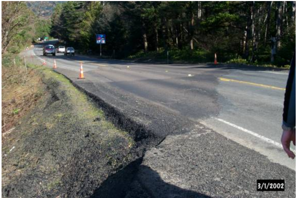
Figure 1: Johnson Creek Landslide on Highway 101
